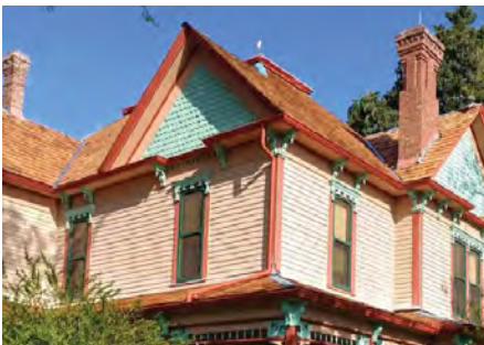
Repair of the wooden shingle roofing on the Ammie Wilson House is an example of typical repairs covered by the National Trust insurance policy.
